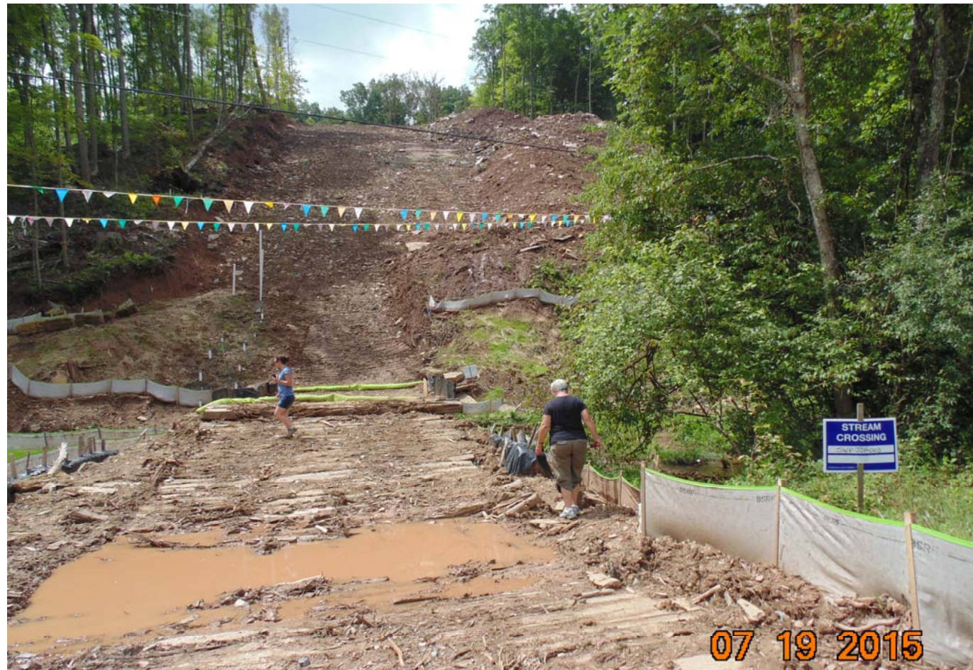
Photo: Stream crossing at Stonewall Gathering Pipeline construction site about 2 miles west of I-79 in central Lewis County, WV. Photo taken on July 19, 2015. The Stonewall Gathering is a 36-inch natural gas pipeline. Much of the erosion and sediment control fencing was failing, and mud was sliding directly into a stream called Sand Fork, about 3/4 mile northwest of an EQT hydrofracking well site.
